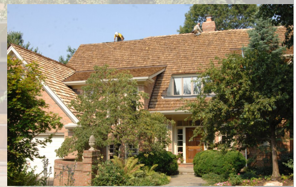
A crew works to complete one of 32 units that were part of the two Trillium phases.
